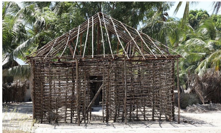
Fig 1. Traditional mud hut (wattle and daub) construction seen in Mtwara, Tanzania. Once the woven lattice of sticks (wattle) is completed, the gaps are filled and plastered (daubed) with sticky mud and stones (photo by Lorenz von Seidlein).
